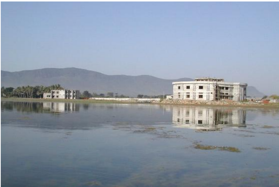
View of wetland education and research centre and residential facility for researchers (under construction)
